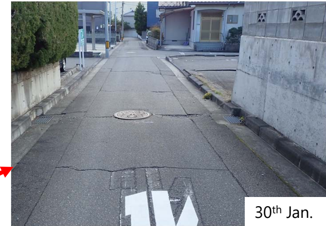
Upper part of the slope: Open cracks
