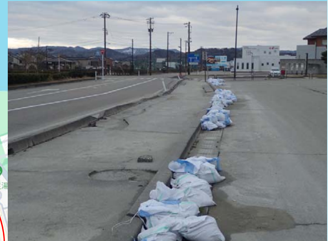
A lot of ejected sand in parking lot
