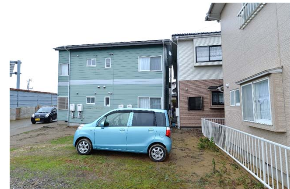
Leaning and settlement of the house (3 rd Jan.)
