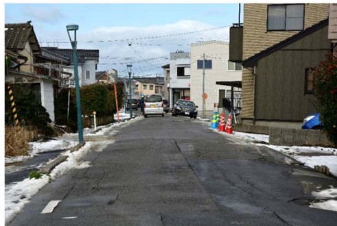
Upheaval of the road (3 rd Jan.)
