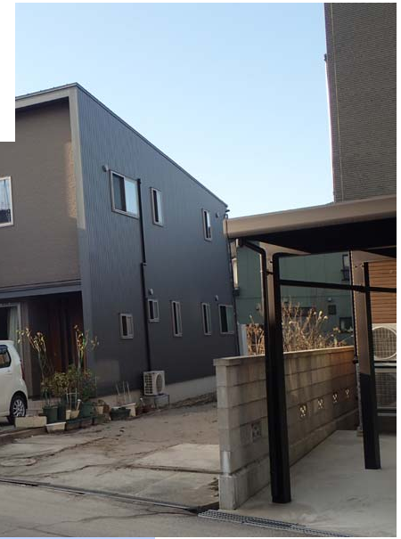
Leaning of house
