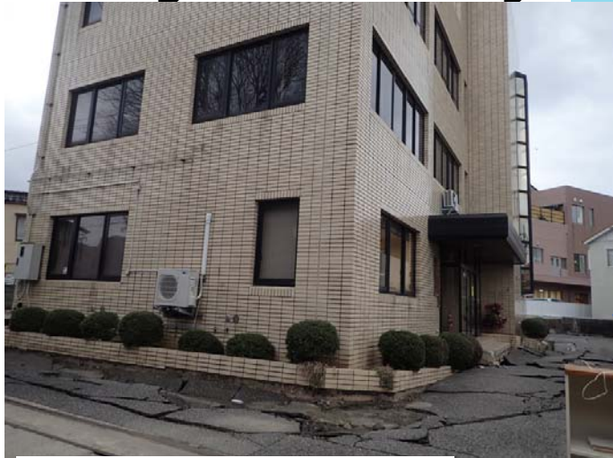
Leaning and settlement
